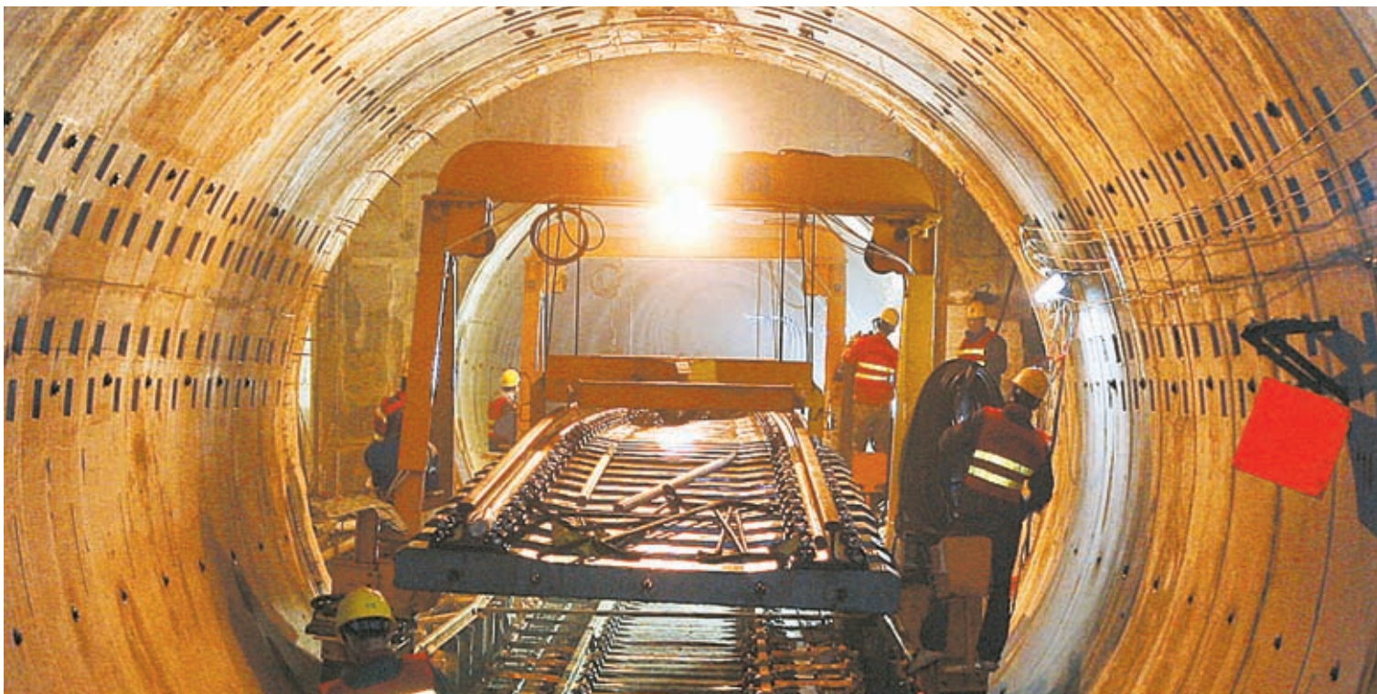
On March 1, 2012, the tunnel for Phase 1 of Metro Line 13 was linked. Since May 28, 1993, when Metro Line 1 launched its trial operation, Shanghai Metro has expanded to 831 kilometers. — Zhang Suoqing
